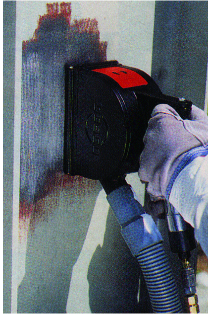
Fig. 2: Rotary impact tool in use on vertical surface, with dust collector attachment
